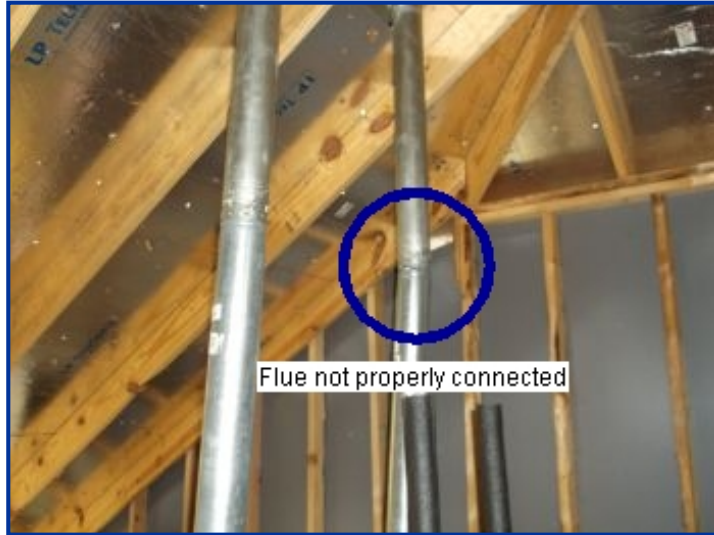
Right side water heater flue
