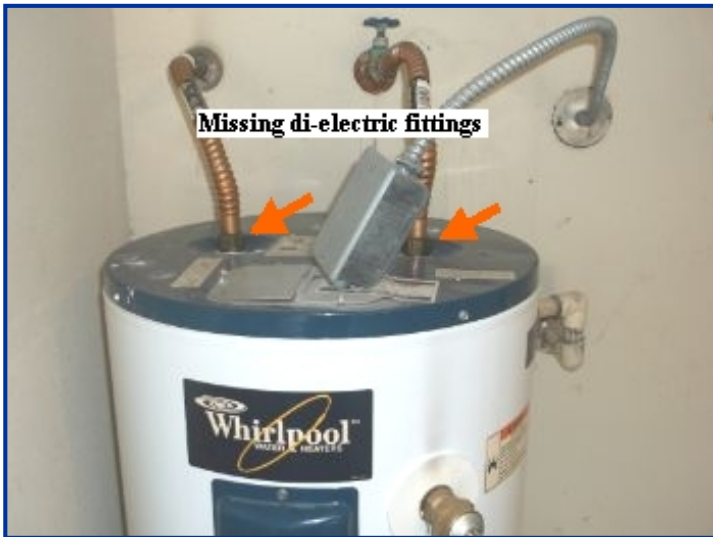
Water heater supply/discharge lines
