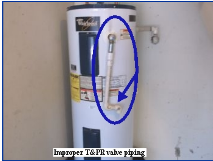
Water heater in garage
